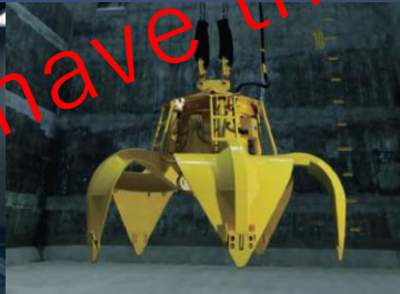
Waste pit/ Waste Crane
